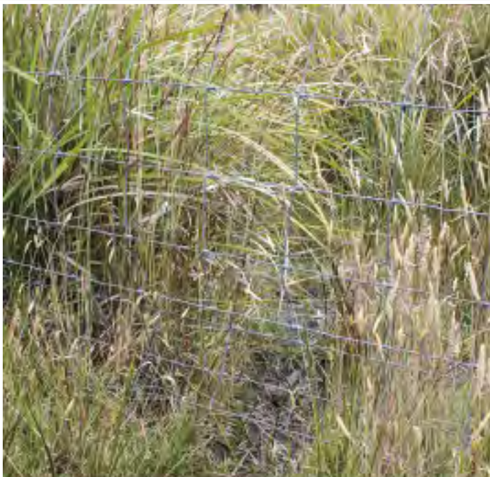
Fence concertina in an early hinge joint mesh fence caused by animal pressure when posts are too widely spaced, Redpa (Steve Pilkington)
